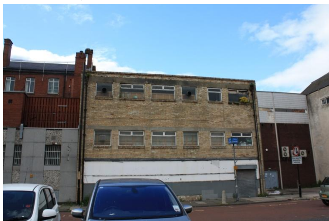
Photograph 4—Buildings on East Street to be demolished showing modern brick construction and flat roofs
